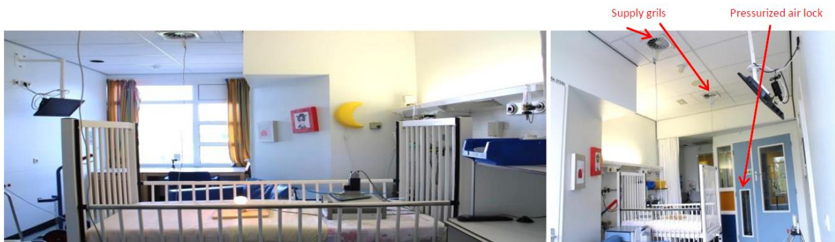
Figure 5 – Isolation room (type 2) at the medium care/high care (MC/HC) department, provided with a pressurized air lock.
