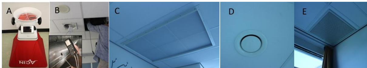
Figure 8 – a) Flow finder and b) Pitot tube for measurement of: c) Air supply, d) Exhaust and e) Recirculation and exhaust grills.
